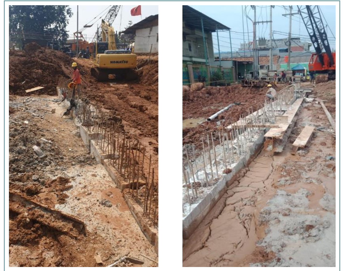
4. Panel DW terpasang
